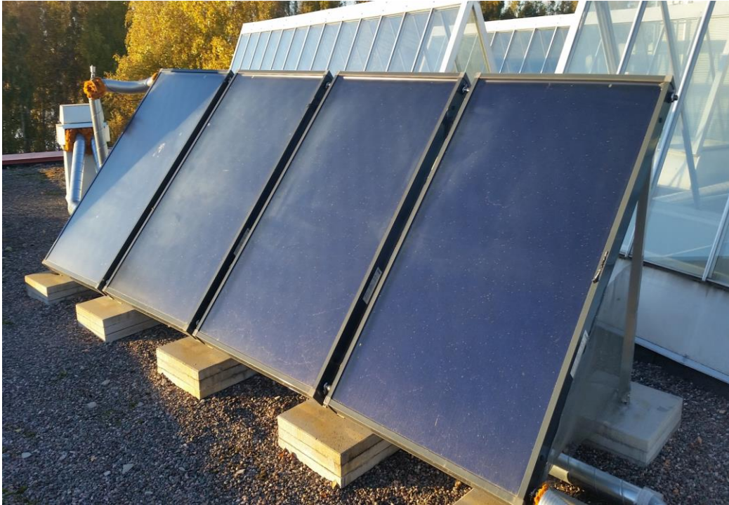
Figure 14 Flat-plate solar collectors on the roof of the building where nZEB laboratory is located.
