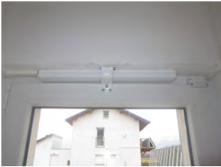
Automatism for windows opening/closing.
