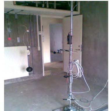
Air, globe and surface temperature sensors, humidity sensors, lux sensor and heat flux sensor in one side-by-side room in EnergyFlexLab.
