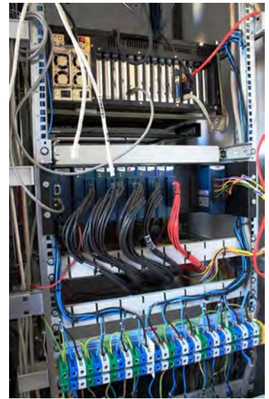
Wiring and connections
