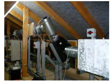
Innovative system of mechanical ventilation in the house attic.
