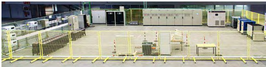
Figure 4: Micro Grid (part of DerLab) installed in TECNALIA-Sustainable Division
