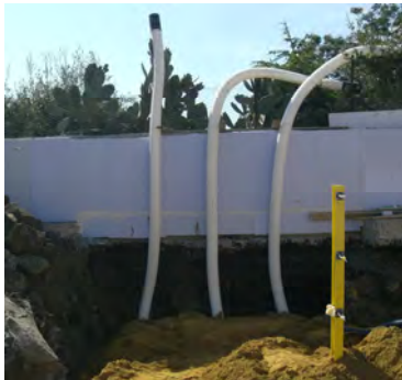
Earth to Air Heat Exchanger here in phase of construction (3 tubes, 10 m long each, 3 m deep). It was designed by eERG-PoliMI in order to maximize energy performances and to have a good layout for monitoring it.
