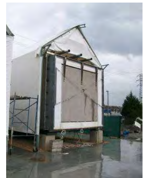
Sample installed in EGUZKI.
