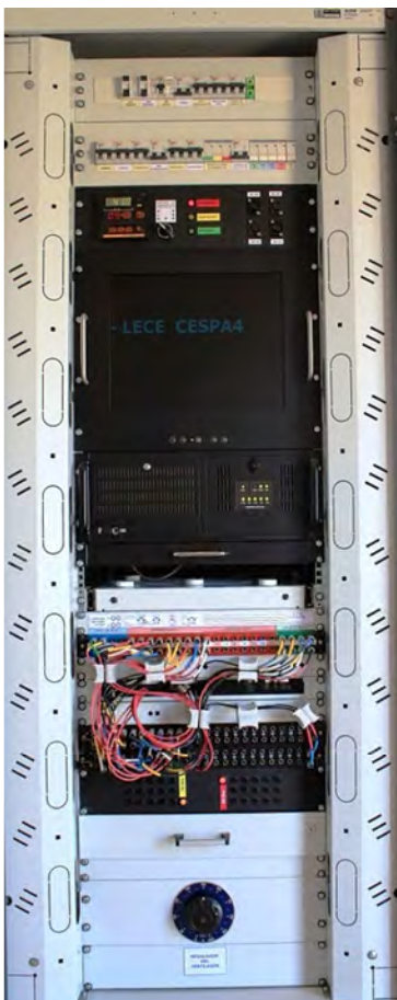
Data Acquisition and Control System
