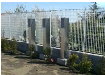
Inlet ducts of Earth to Air Heat Exchanger
