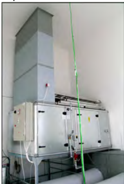
Ventilation system in the experiment room
