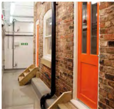
The Energy House and its adjacent conditioning void, used to control and monitor energy loss and heat transfer through party walls.
