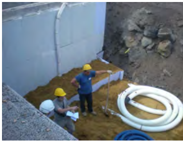
Earth to Air Heat Exchanger here in phase of construction (3 tubes, 10 m long each, 3 m deep). It was designed by eERG-PoliMI in order to maximize energy performances and to have a good layout for monitoring it.
