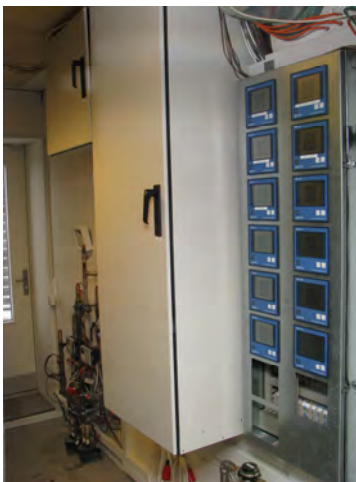
Heat meters at EnergyFlexLab.
