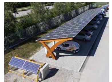
Electrical cars and solar station.
