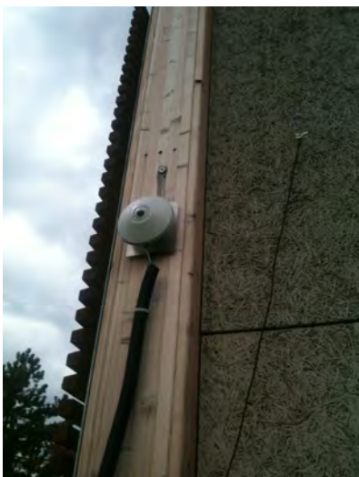
The pyranometer device to measure the global vertical solar radiation on test wall.
