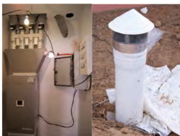
Heat Pump and Ground heat exchanger
