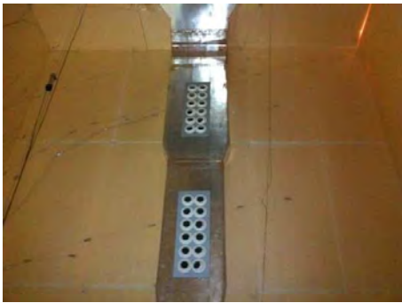
Figure 4. HVAC system. Air distribution system
