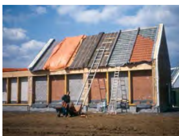
Picture during construction of building elements: the measurement bays with fill in masonry for test walls and the construction of test roofs are visible.
