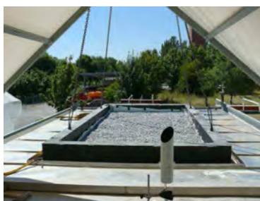
ILARGI: installing the roof covered by gravel to be tested inside the frame.
