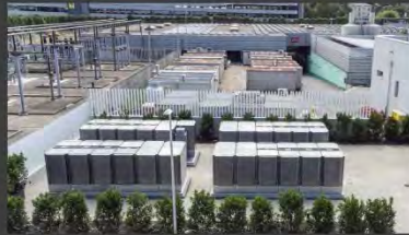
Ferrari, Maranello, Italy Packaged Energy Server
