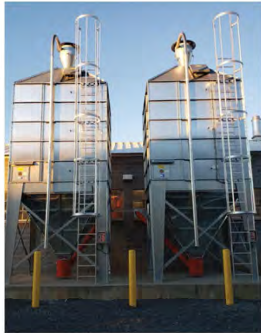
This Centralized Biomass Pellet Silo in Umatilla, Oregon, is an Oregon Army National Guard renewable energy project with a resiliency component which uses biomass from local forests for heating several buildings. (Photo Credit: U.S. Army)
