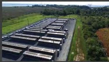
Delmarva Power, Delaware Utility Installation
