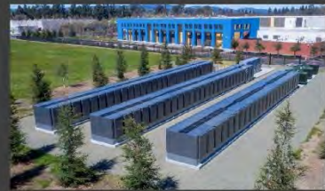
Kaiser Data Center, Napa, CA Data Center Installation
