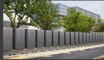
Intel, Bangalore, India Microgrid Installation
