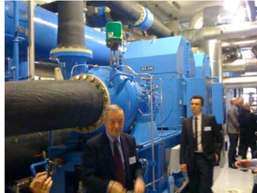
Large heat pumps ....
